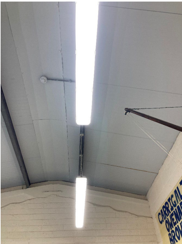
LED Lighting in Preschool Classroom
