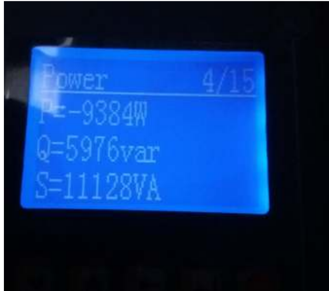
Photo 1. New Building Sub Meter - Showing ca. 9.3kW (continue to read this meter to separate out consumption)
