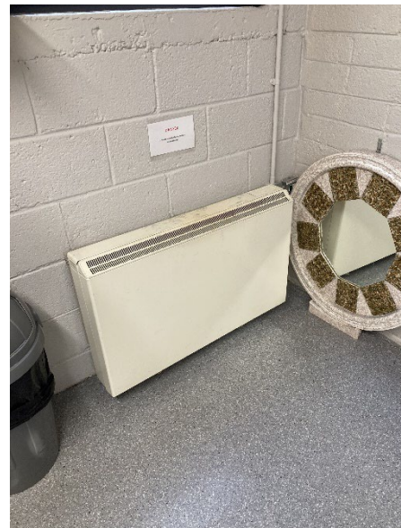
Storage Heater in Kitchen
