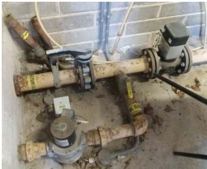
Photo 2 – Gas inlet point to boiler room. - Some tidying up required
